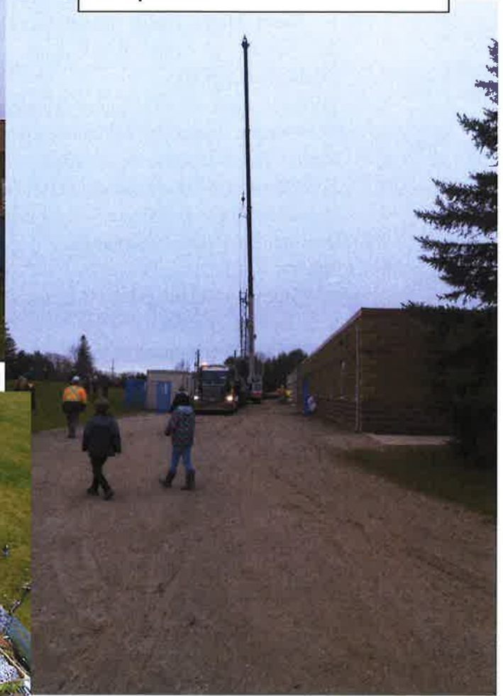
The students were given the opportunity to see the roof trusses being laid! What an experience!
